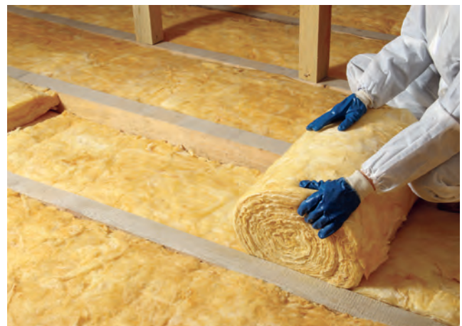
▲ Figure 3.4 Loft insulation
